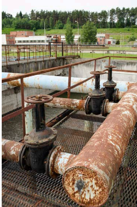
Photo Caption: Corrosion at a standard water facility. Corrosion factors were significantly more intense at the Carlsbad Reverse Osmosis Desalination
